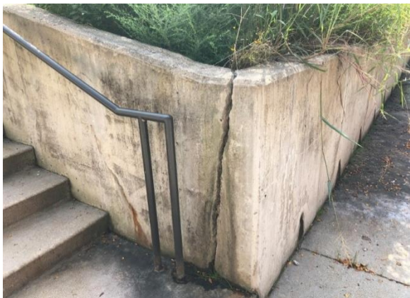
Cracks at Retaining Wall
