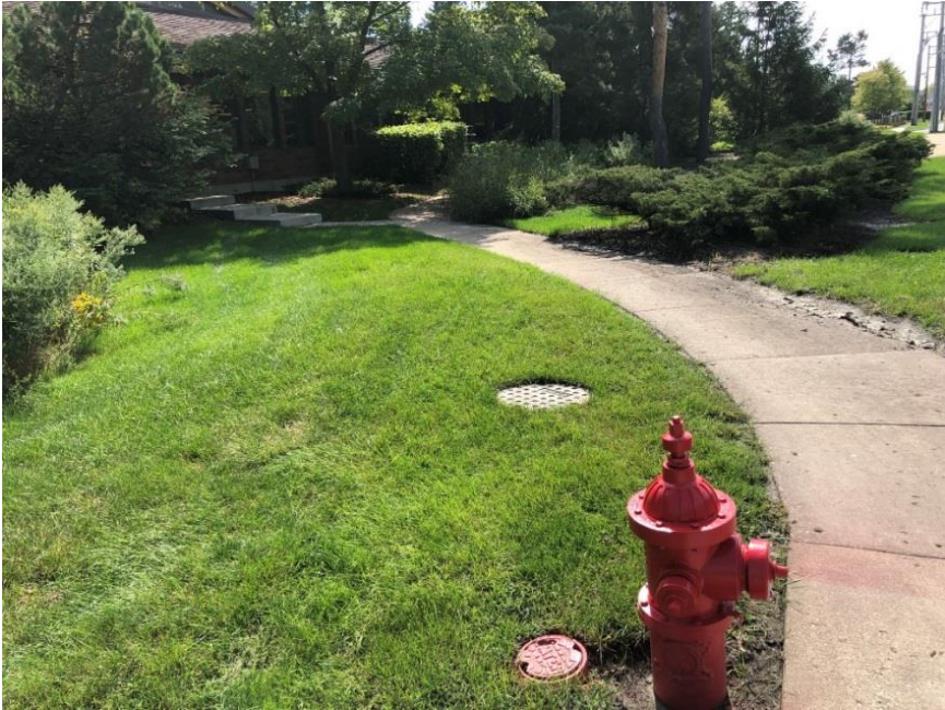
Figure 7: Area of Flooding at South Sidewalk
