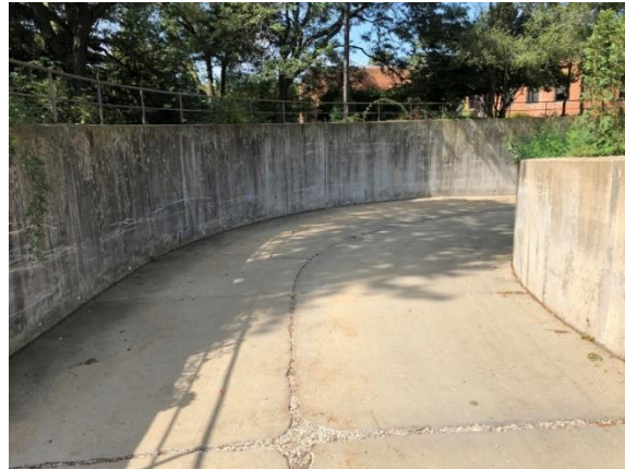
Figure 2: Pavement cracks at Service Drive
