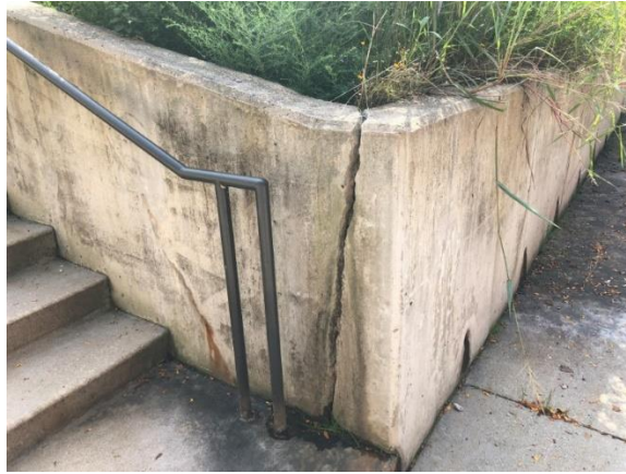
Figure 5: Cracks at Retaining Wall
