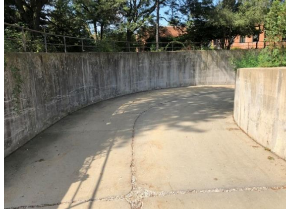
Pavement cracks at Service Drive
