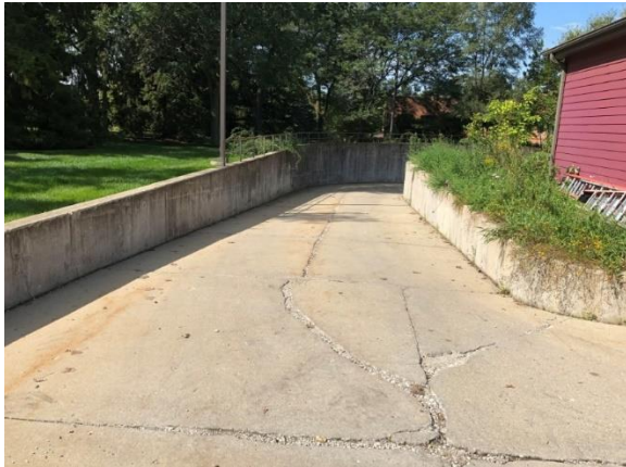
Figure 1: Pavement cracks at Service Drive
