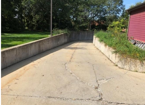
Pavement cracks at Service Drive
