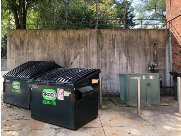
Figure 4: Cracks at Retaining Wall
