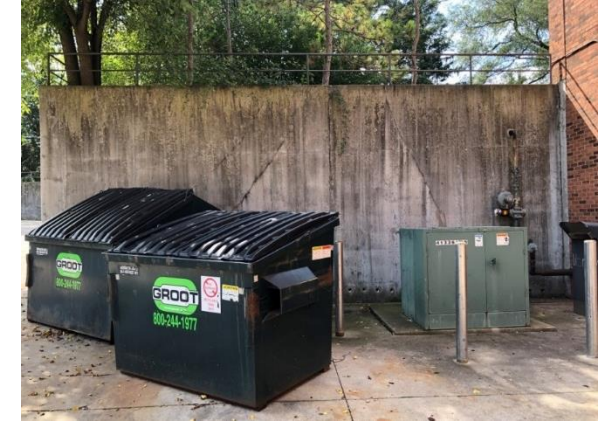
Cracks at Retaining Wall
