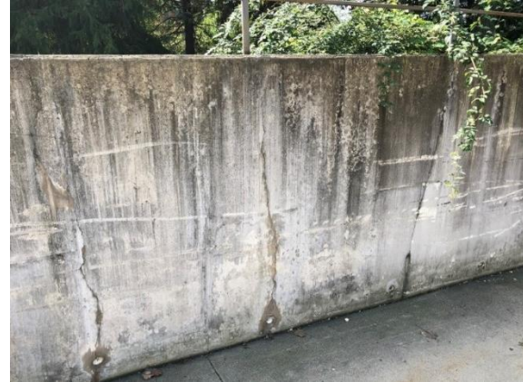
Cracks at Retaining Wall
