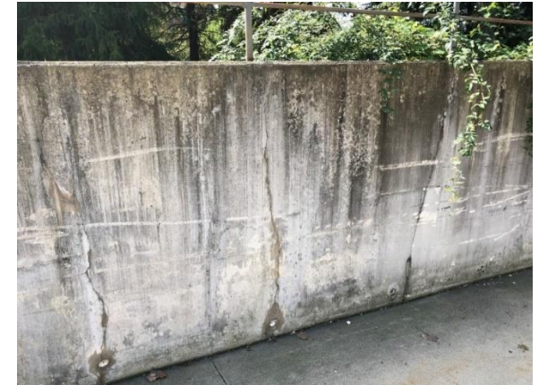
Figure 3: Cracks at Retaining Wall
