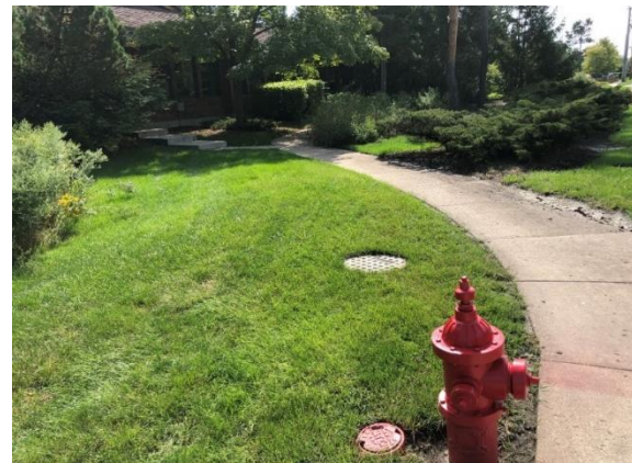
Area of Flooding at South Sidewalk
